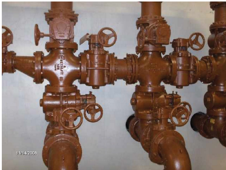
FIGURE 7. Pipe Gallery in Treatment Plant in Morris, IL
