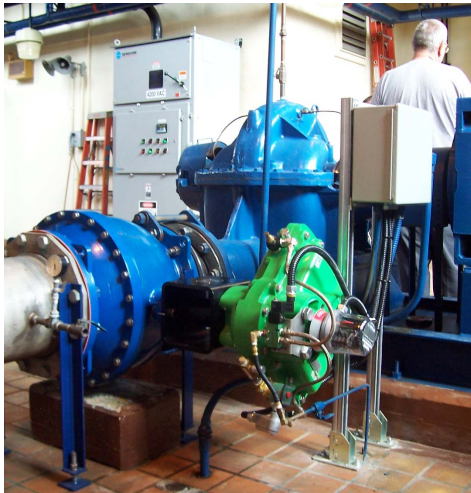
FIGURE 1. Pump Control Ball Valves in Ohio, USA
