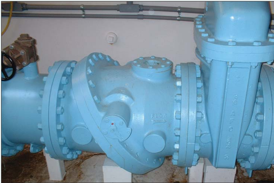
A tilted-disc check valve often provides slam-free operation without dashpots because of its short stroke and balanced disc.
