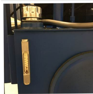
Figure 5. Sump Tank Sight Glass
