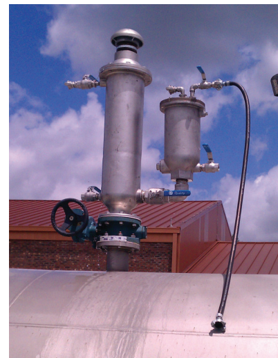
Lithia Water Treatment Plant Tampa, FL
