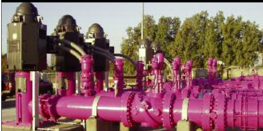
Figure 2. Air valves on pump discharge reduce air in pipelines in Chino, CA.
