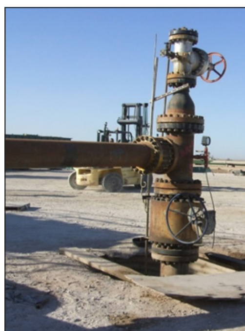
Figure 3. 16 NPS Class 600 QuadroSphere® 16-3/4 in. Bore Brine Well Master Valve at Wellhead
