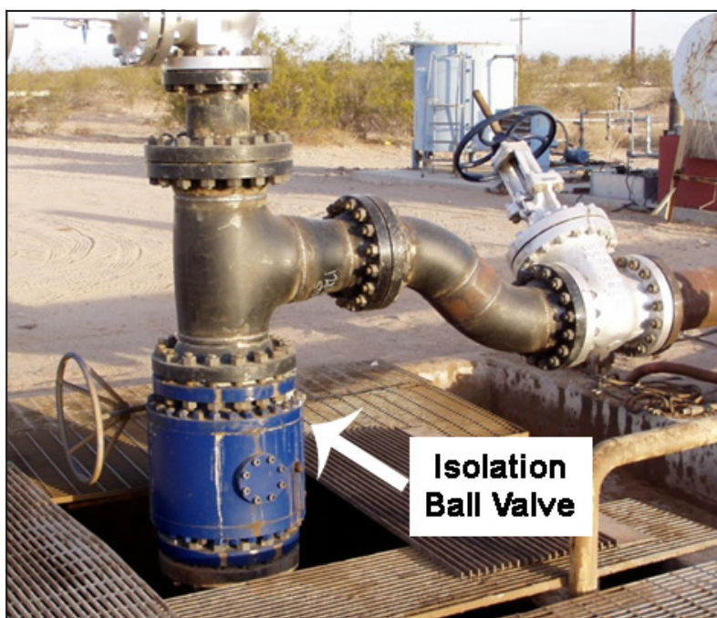
Figure 2. QuadroSphere® Ball Valve at Wellhead
