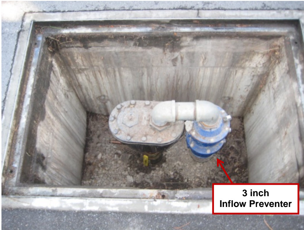
Figure 6. Air Valve Vault, Foster City, CA
