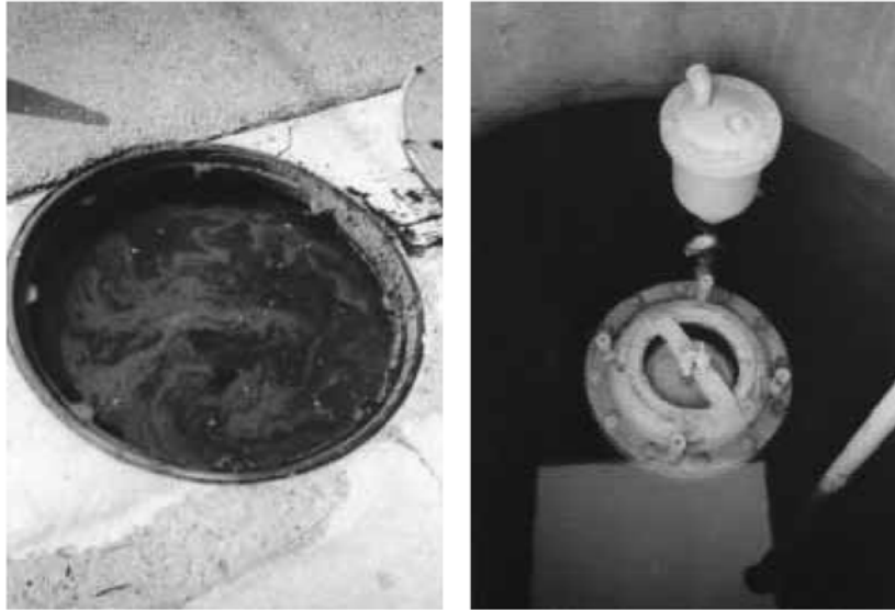
Figure 1. Submerged Air Valve Vault [LeChevallier]
