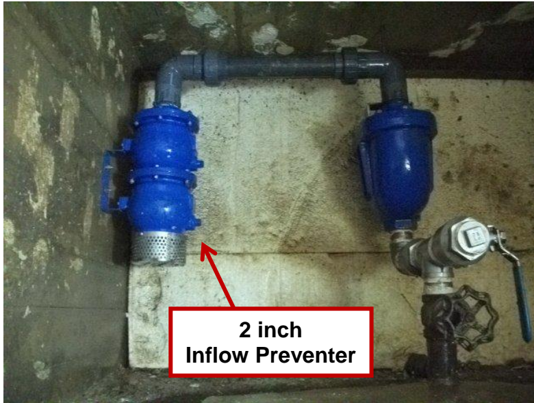
Figure 8. Air Valve and Wall-mounted Inflow Preventer, Region of Peel, Canada
